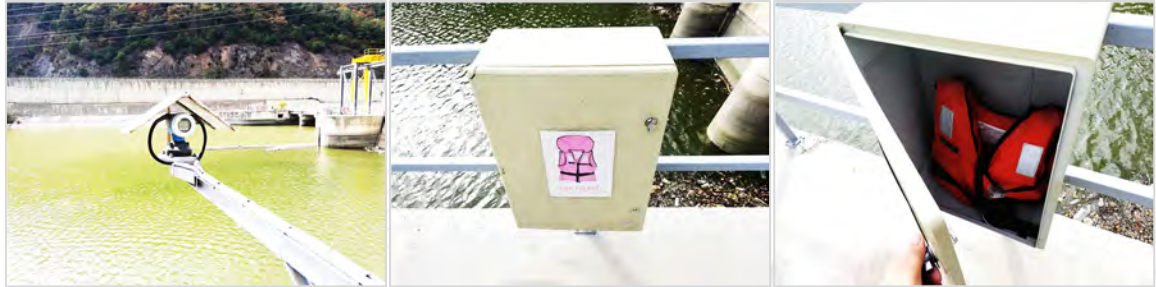
Picture 127 DORUK HEPP ELECTRICITY WARNING SIGN, FENCE OF GRID AREA AND CCTV SYSTEM VISUALS
