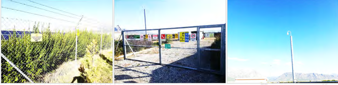
Picture131 OMİCRON & PSİ SEPP TRANSFORMER HOUSE, FENCE APPLICATION, CCTV SYSTEM AND EXTERNAL LIGHTING VISUALS
