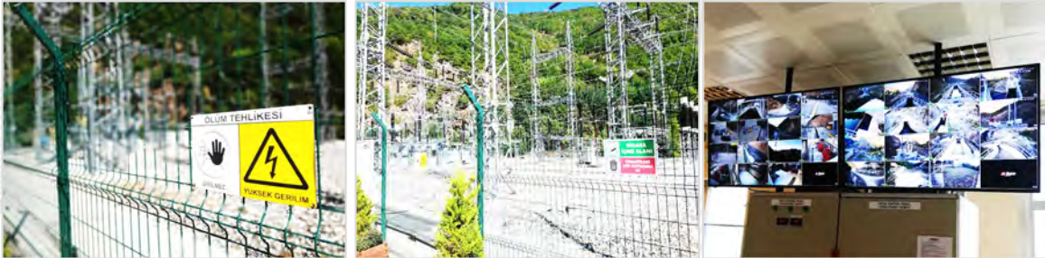
Picture 128 ÜÇPINAR WEPP FENCE, WARNING SIGNS (CAUTION FALLING ICE, ELECTROCUTION RISK)
