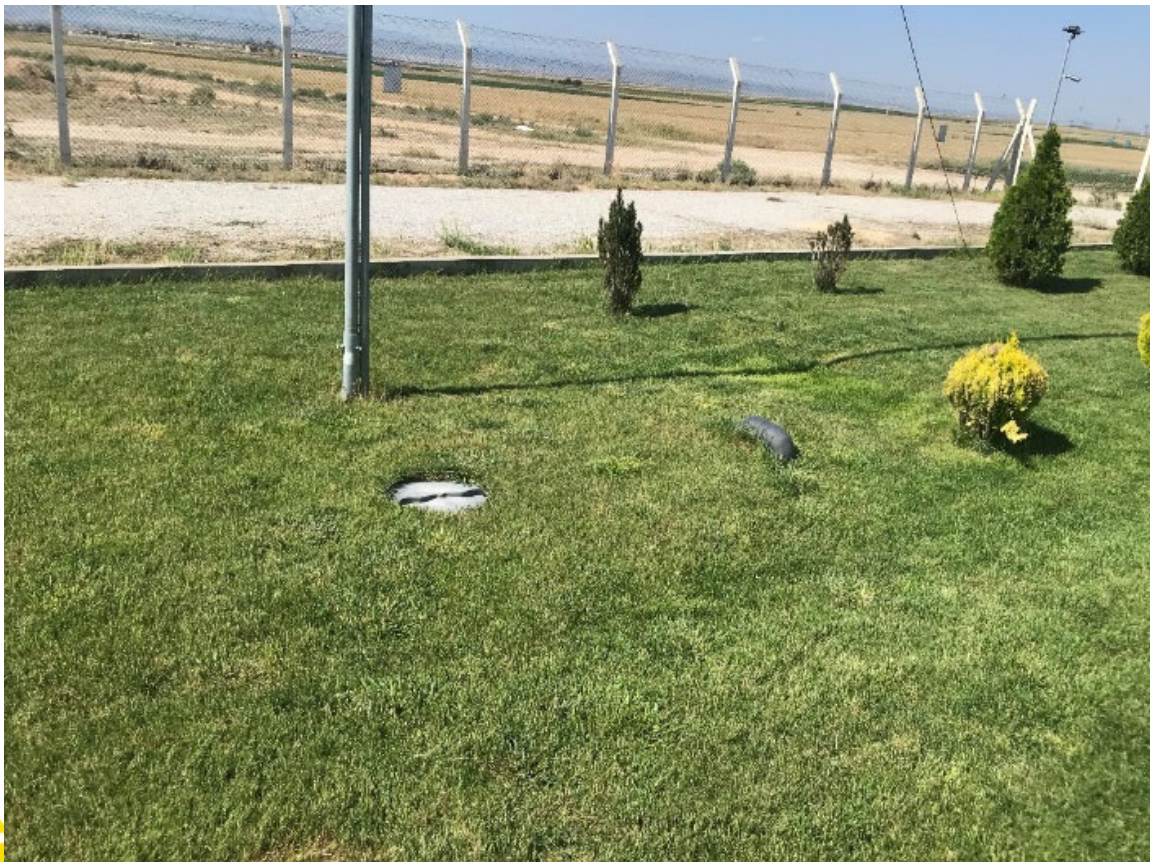
Picture 61. EXAMPLE OF SEPTIC TANK FIELD FOR ME-SE SPP
