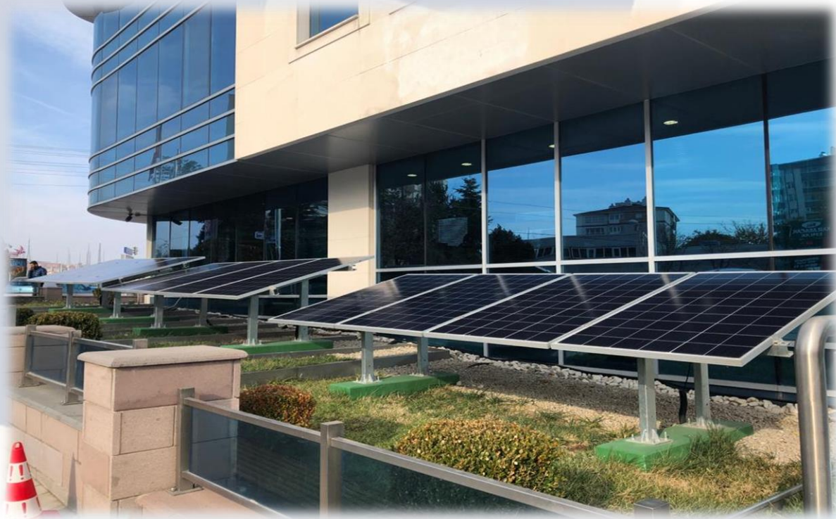
Photograph 91- Head Office Off-Grid System
