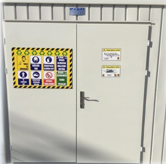
Hasanoba WPP-Warning Signs
