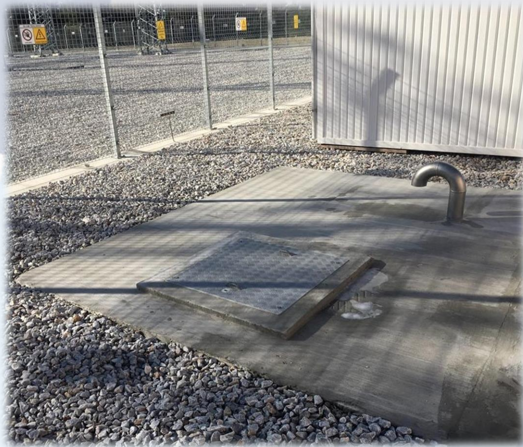
Photograph 90- Hasanoba WPP Leakproof Septic Tank
