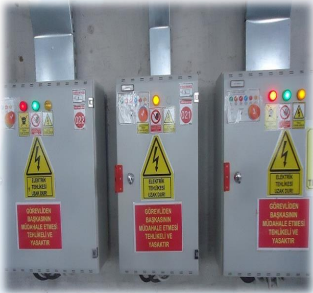
Demirciler HEPP-Warning Signs
